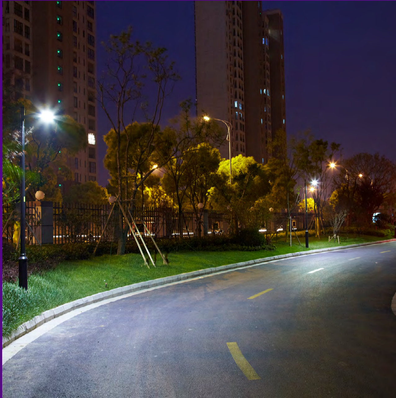
Lighting for residential and connecting roads
